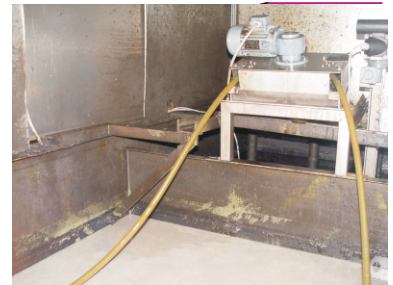
Oil skimmer model W40 at waste water tank
