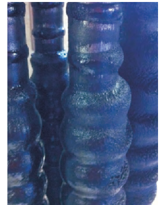
Ferritic particles on magnetic filter rods
